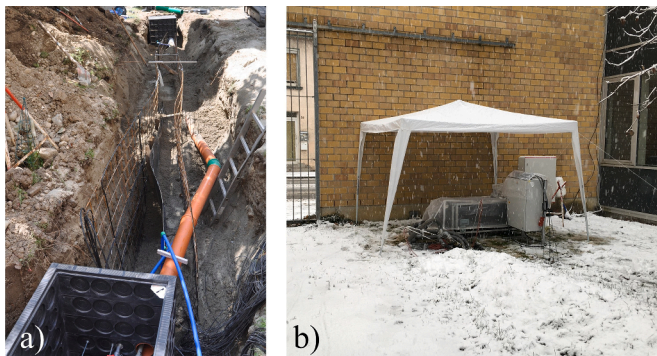
Fig. 5. a) Trench collector and measurement equipment during installation, b) thermal response test device attached to the trench collector plant at the experimental site.
